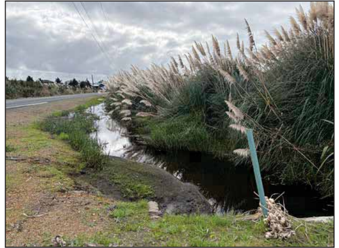
The deep water filled drains alongside Marsden Bay Drive
