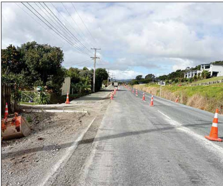
The Wharehine crew is now concentrating on building the shared trail linking section alongside the road.
